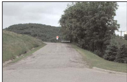
figure 3.5 Existing S. Chestnut street ramp to become multi-use path for cyclists and pedestrians
